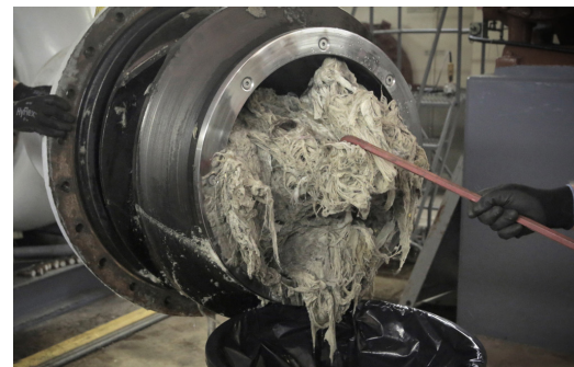
Picture shows a pipe clogged with wipes being cleaned out.
